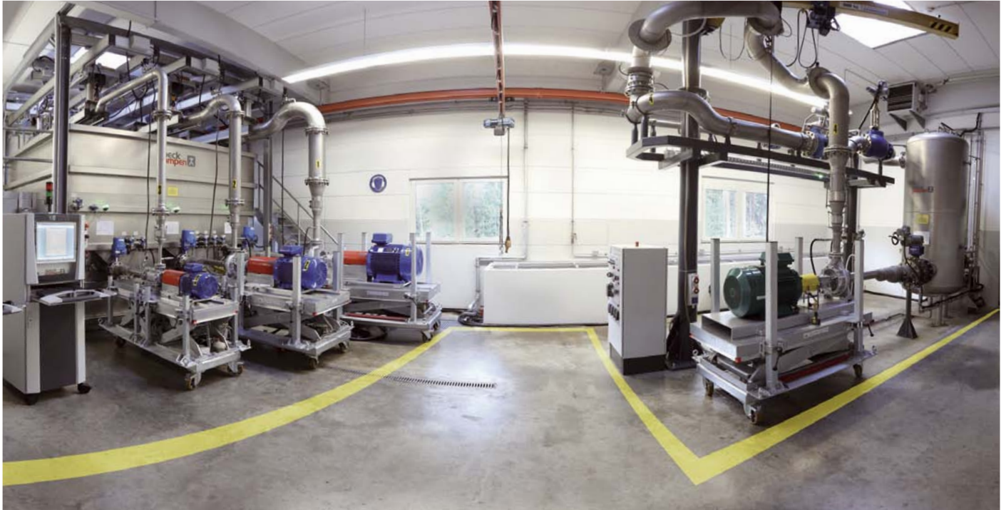
Test stand for liquid pumps on the premises of Speck in Roth Measuring of hydraulics, power requirements, axial thrust, vibrations and NPSH values. Heads of up to 400 m and flow rates of up to 750 m 3 /h.
